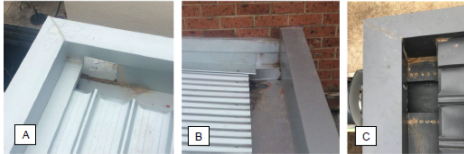
Image 1: Examples of non-DtS box gutter installations
